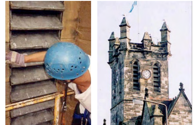
Louvre replaced on a listed building with radio transparent replica Photographs courtesy of Dynamic Concepts
