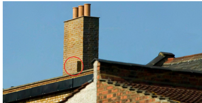
Good example of disguised equipment
